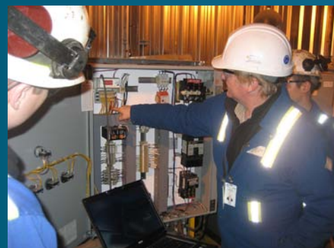
Summit provides start-up services and HPU training on how to setup and maintain your system.
