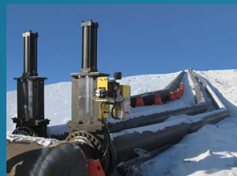
Field installation in an outdoor cold weather environment.
